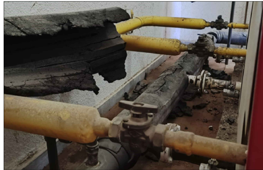
SUBMINISTRAMENT DE GAS NATURAL A CALDERES MODULARS
